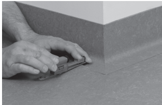
Cut out the floor covering that will be laid on top of the skirting
